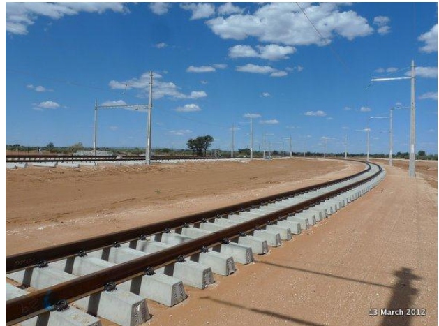
Tshipi Borwa - Rail siding
