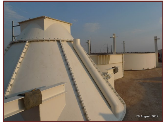
Tshipi Borwa – Rapid load-out station components
