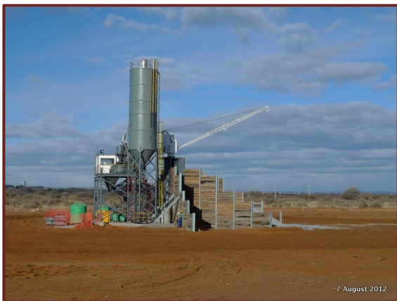
Tshipi Borwa – Concrete batch plant
