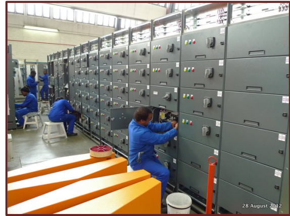
Tshipi Borwa – Low voltage panels assembled
