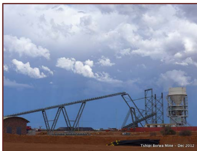
Figure 21 – Tshipi Borwa Rapid Load-Out Station and Feeding Conveyors
